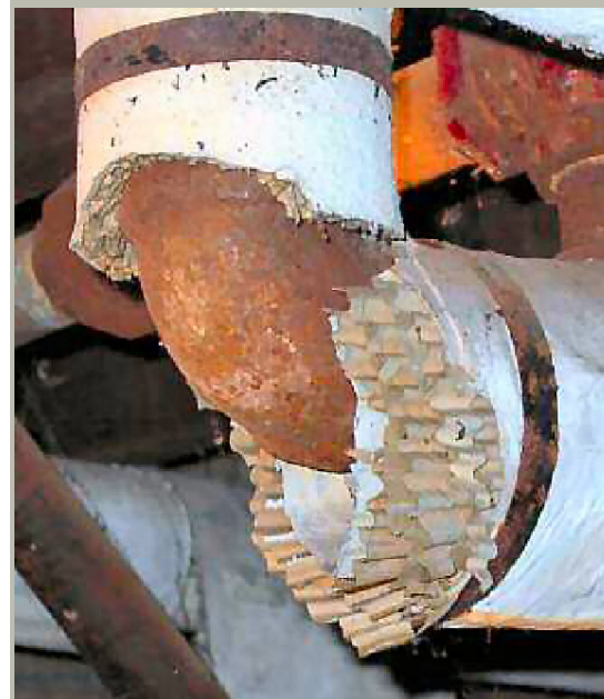
Damaged asbestos pipe insulation.
